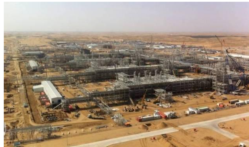
South Yoloten gas field development, Turkmenistan
